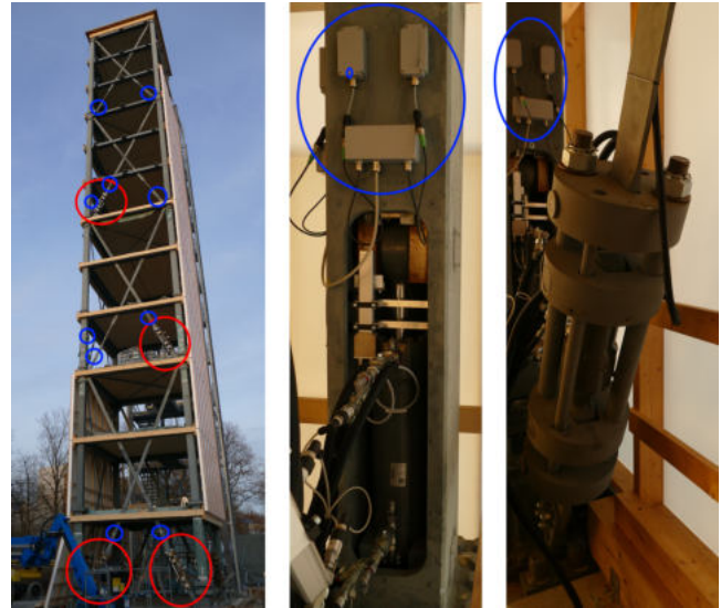
Fig. 1. Left: adaptive high-rise structure D1244 during construction with hydraulic actuators (red) and sensors as strain gauges, camera-tracked LEDs, etc. (blue). Middle and right: close-up of actuator in vertical column and diagonal bracing, respectively.
